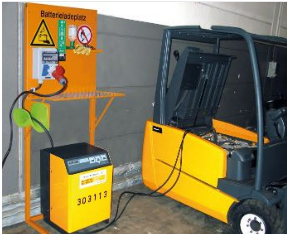
BL with CEEform socket 400 V charging the battery of an electric forklift truck
